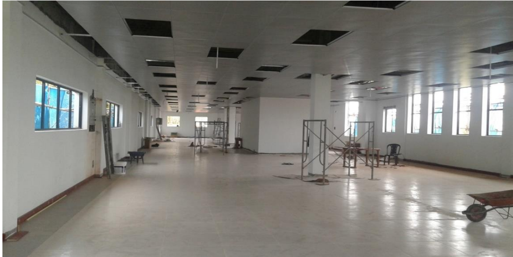
Third floor of the stores complex where construction work has been completed
